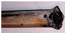
View of the inboard end of the centre aileron push rod from the left wing showing localized heating, part of the fork end fitting and undistorted tube section
